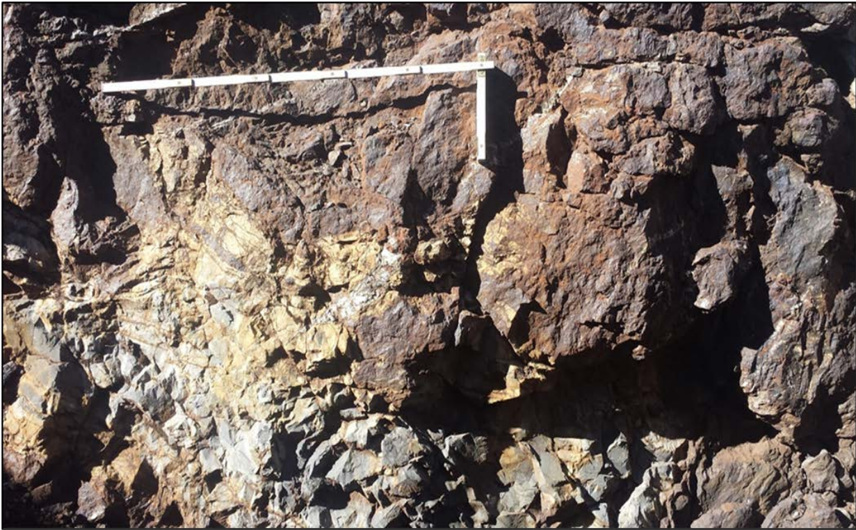
Figure 5: Inside pitted showing looking northwest
