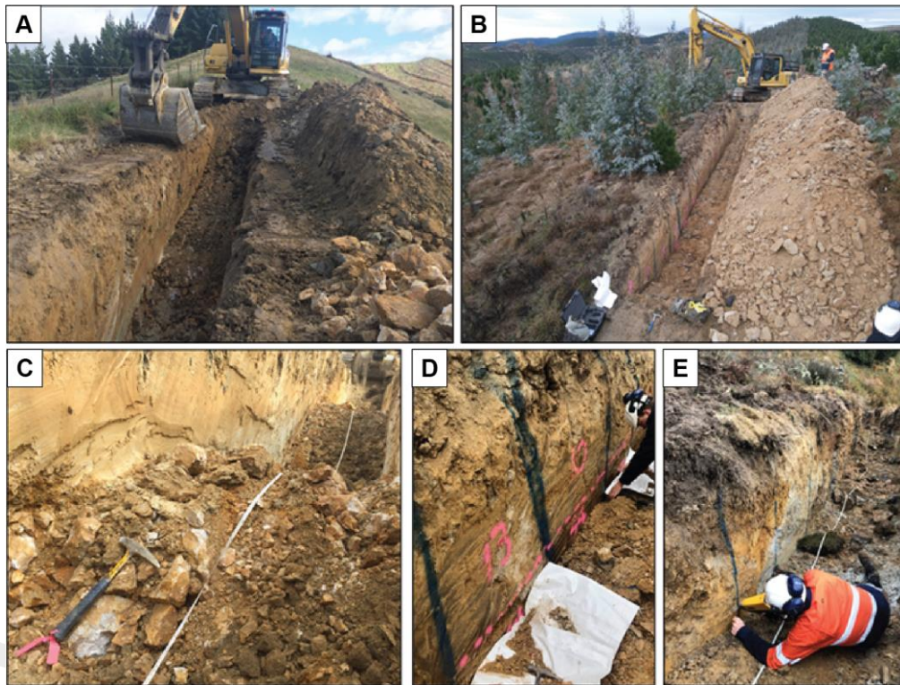
Figure 9-5: Photographs from the trenching campaigns. A) Trench 12 before mark-up; B) Trench 13 after mark-up; C) quartz vein outcrop in Trench 02; D) close-up photograph of the trench mark-up with the tarpaulins laid to collect the sample; E) pXRF analysis of one of the trenches.
