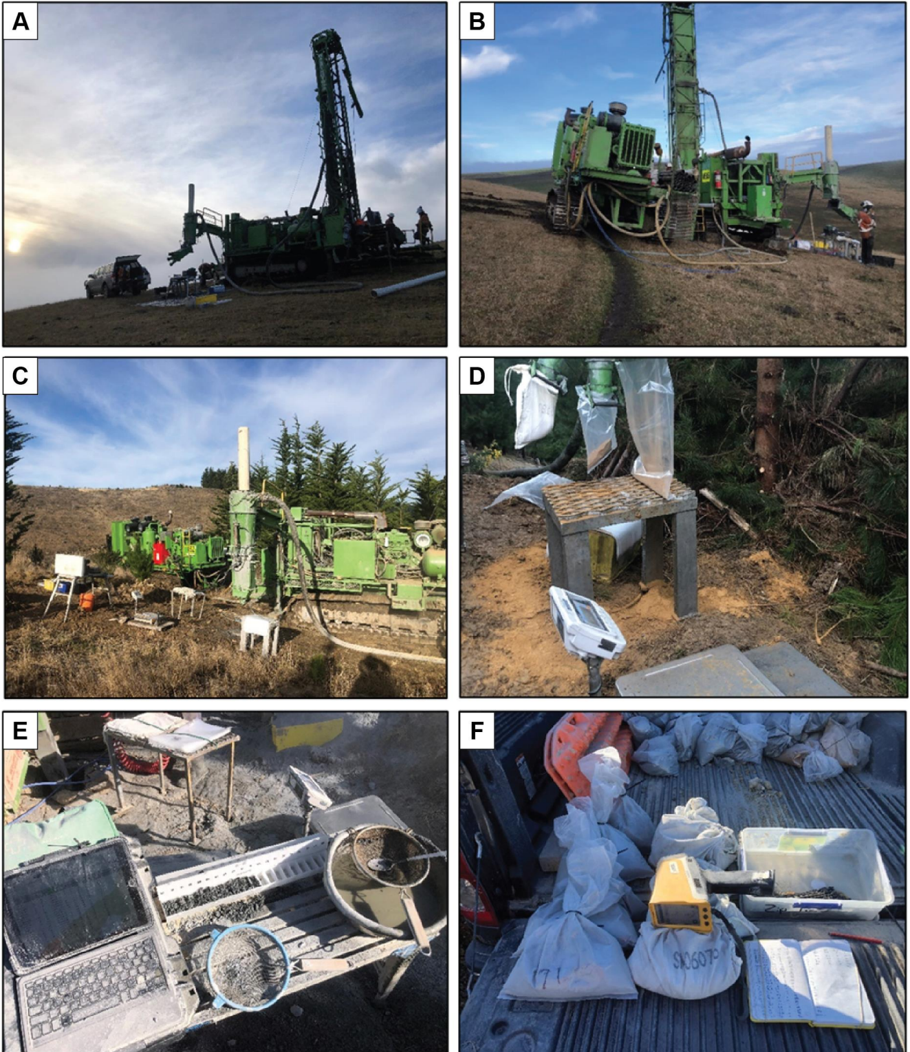
Figure 10-6: A) Photography of the Schramm T660 H Rotadrill drill rig mounted on a CAT325 wide track unit with a Sullair 900cfm x 350 psi air compressor. B) Komatsu CD1 crawler unit with an additional M41 1800 cfm x 870 psi booster assisting the rig. C) View of the sample set-up and rig with a three-tier splitter. D) Splits A, B and C attached to the splitter with scales nearby for weighing samples. E) Logging set up with iPad for recording entered data and chip trays, with wet sieved RC chips. F) Split A and B side by side, post weighing, ready for pXRF analyses and data recording.
