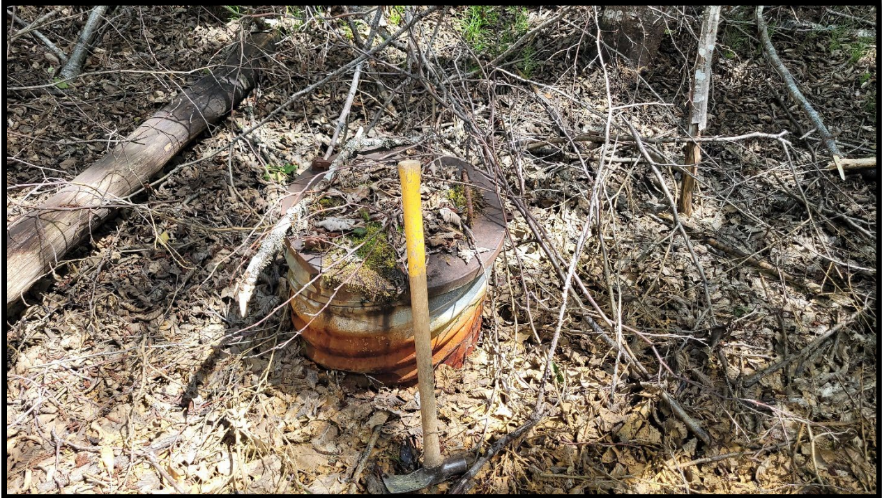
Figure 12-4. Overflow drainage culvert at the lowest elevation of the stored waste and mineralized material from the underground workings (taken June 8, 2024; Station SW24-5, 5414610N, 433603E, NAD 83 Zone 10).
