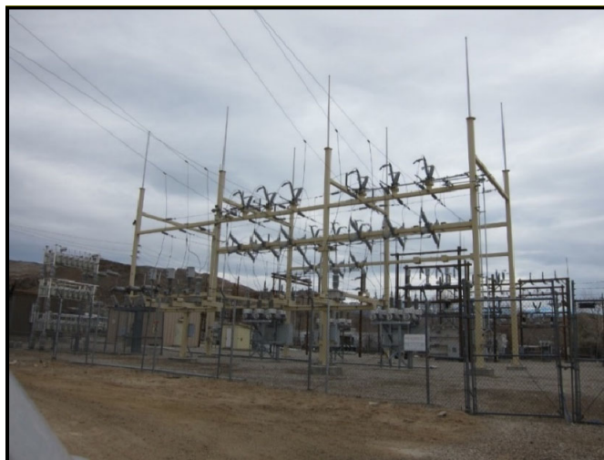
Figure 4. Silver Peak Electrical Substation
