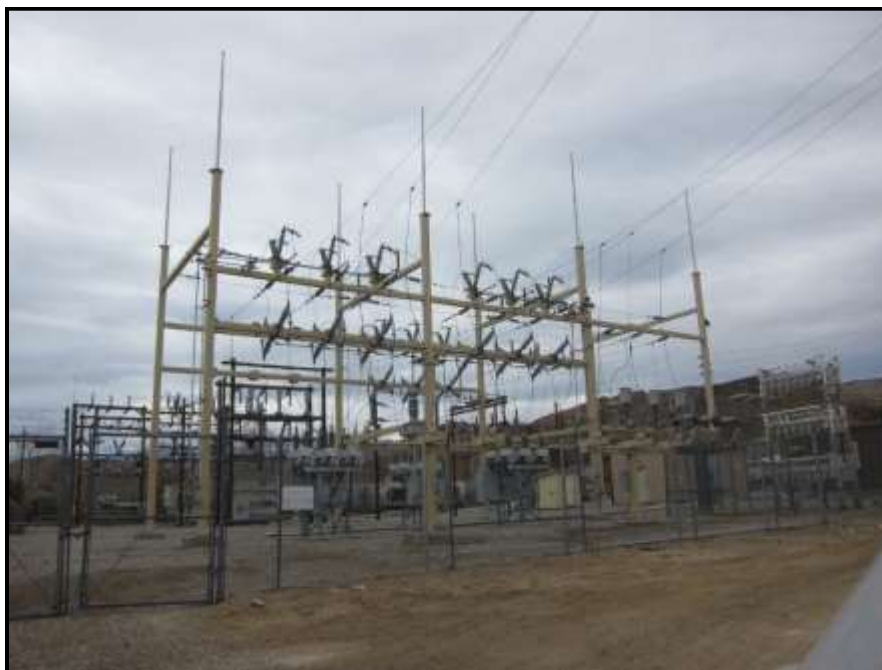
Figure 4. Silver Peak Electrical Substation
