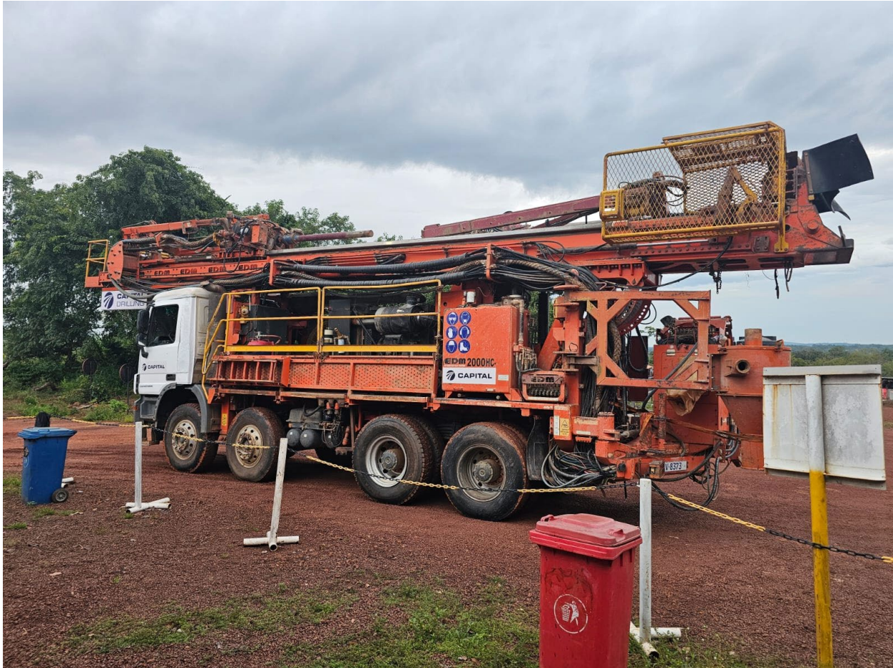
Figure 5: EDM2000HC multi-purpose drill rig mobilizing to the Diguifara project. Photo courtesy of Capital.
