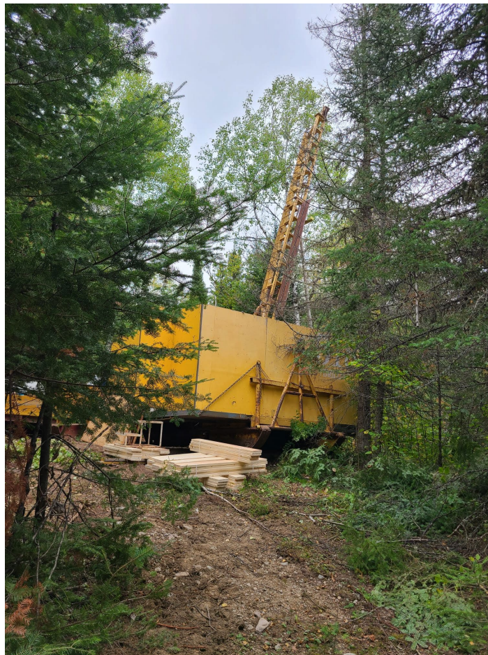
Figure 1. Lining up the drill for the first hole on the South pad.
