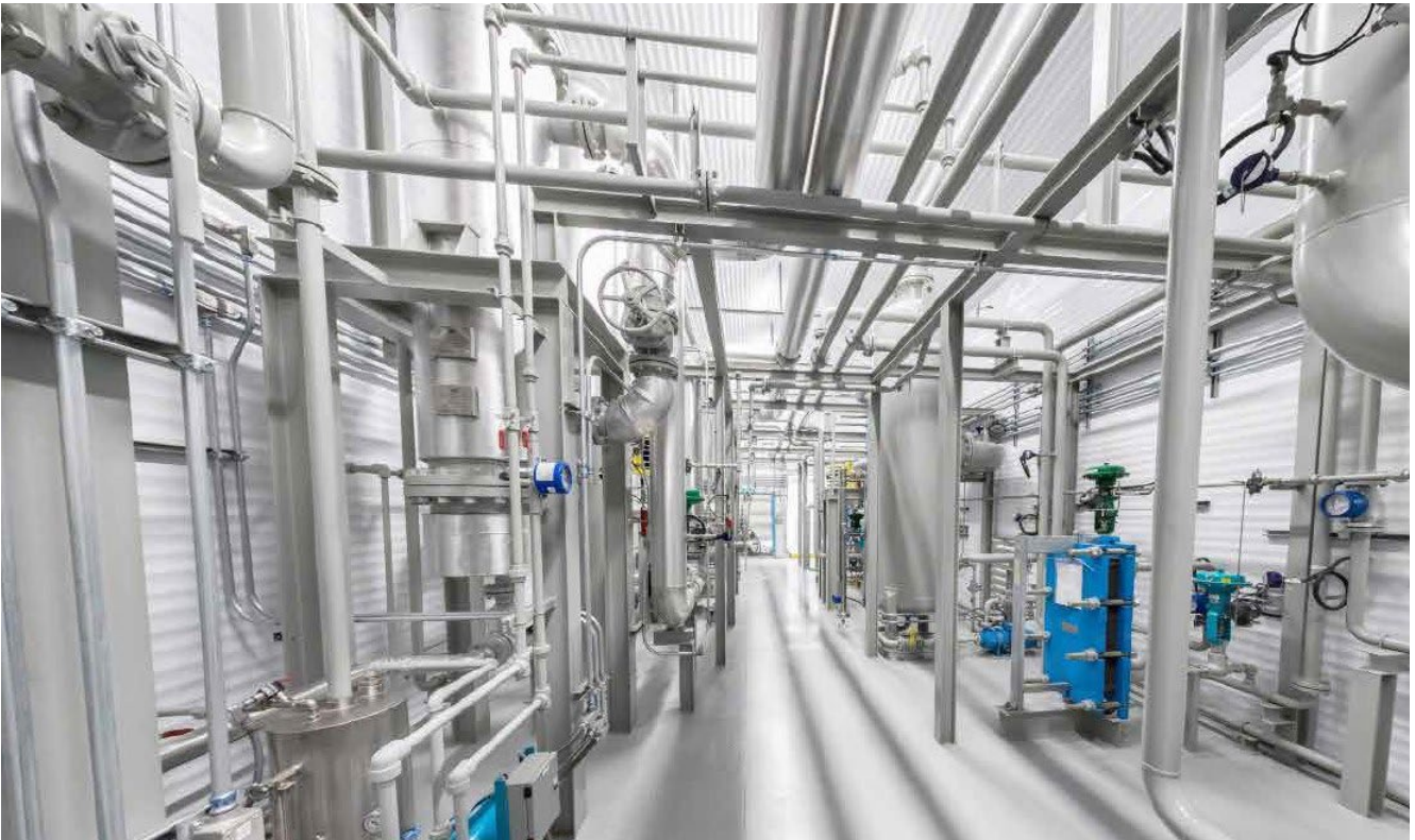
Modular designed CO 2 capture unit. designed by Delta
