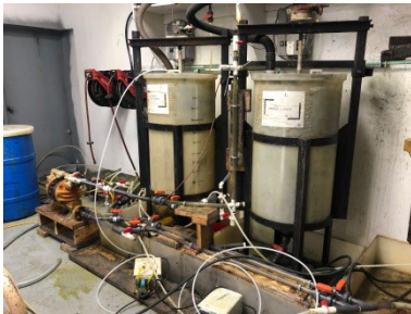
Settling and Flocculation Tanks
