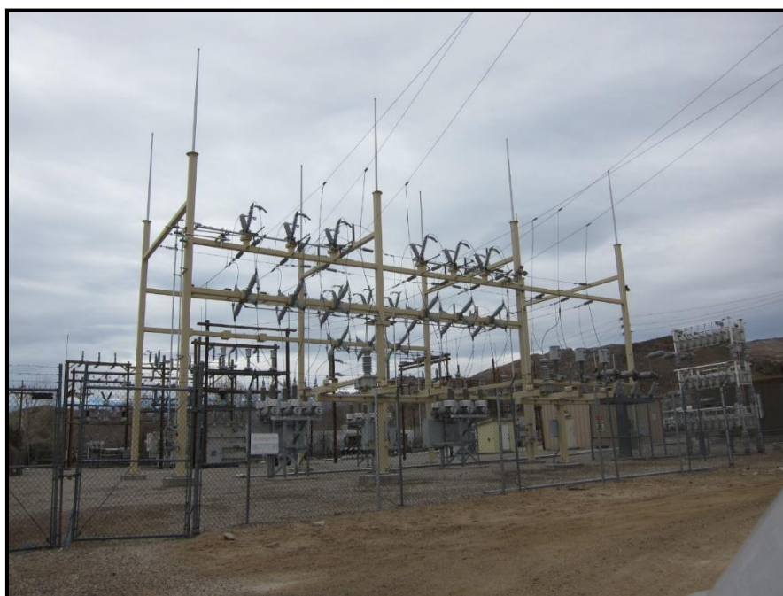
Figure 4. Silver Peak Electrical Substation.
