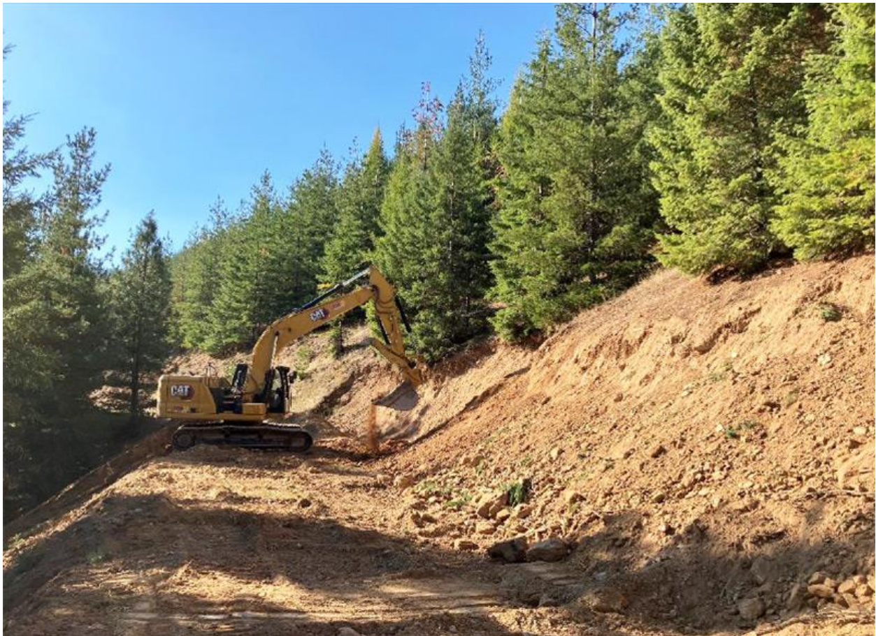
Photo 1: Site preparations underway at Ranger-Page Project to ready for the arrival of the Integri-Core drill rig.
