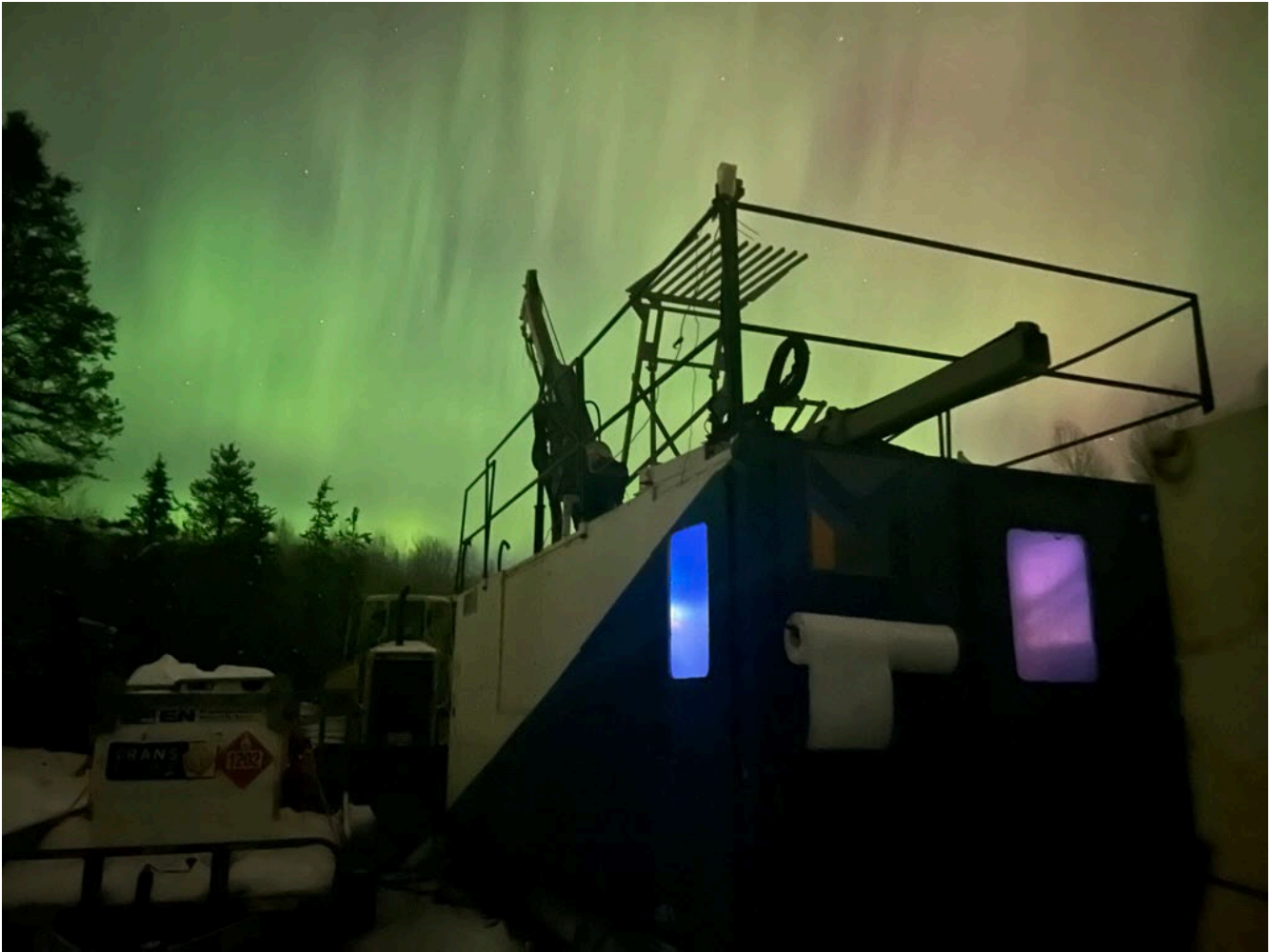
Figure 7: Les Forages Chapais (NB) HTM2500 Deep Surface Drill Rig with Onsite Starlink Internet Support
