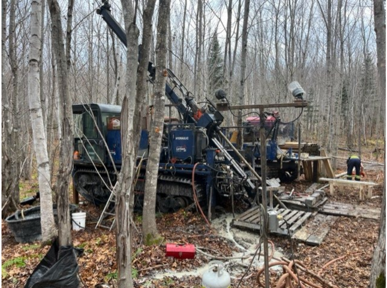
Figure 1: Lantech Trackmounted Drill Rig onsite at California Lake Project, Bathurst Mining Camp, NB
