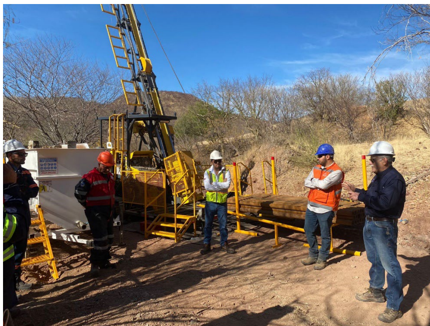
Plate 1. Photo of Core Drilling starting at the Gran Pilar Gold-Silver Project, Sonora, Mexico.
