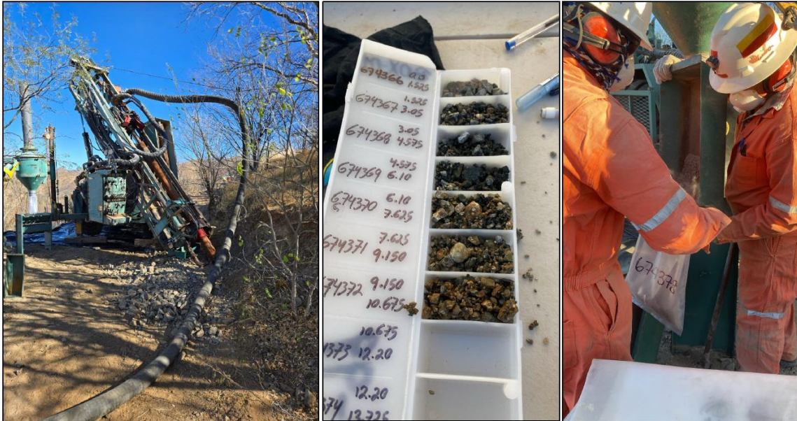
Plate 1. Photos of RC Drilling Restarting at the Gran Pilar Gold-Silver Project, Sonora, Mexico.
