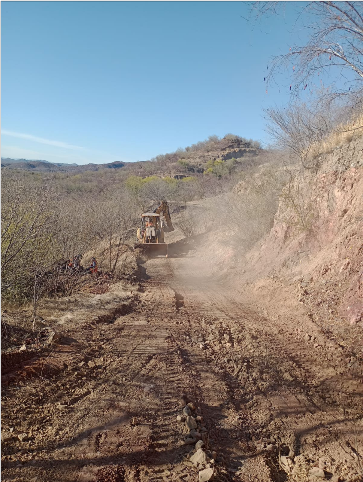
Photo 5. Excavation Prep at Pilar – Main Zone. Recent Channel Sampling Will Guide Bulk Sampling
