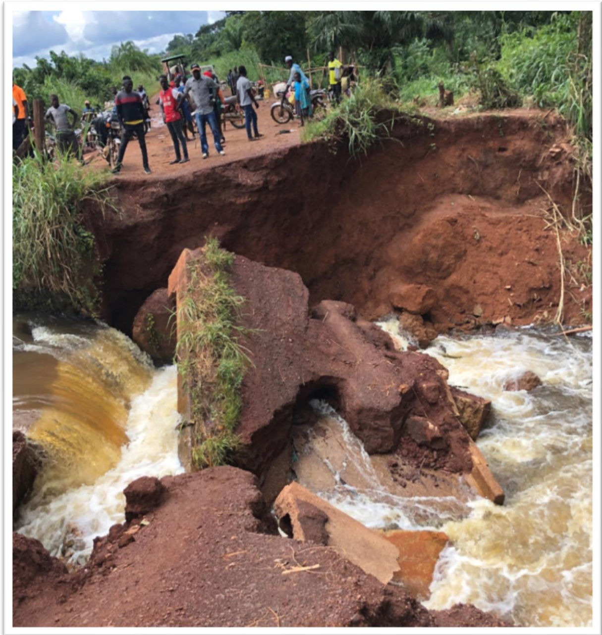
Figure 5.4: Bridge Wash-Out Wanga Village DRC (source Geosure November 2019).
