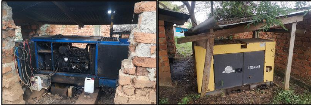
Figure 5-1. Generators observed on the project camp, May 2021.
