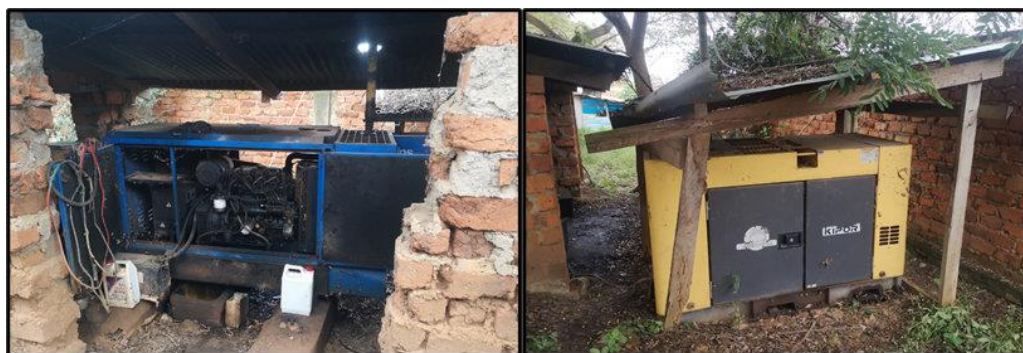
Figure 5-1. Generators observed on the project camp, May 2021.
