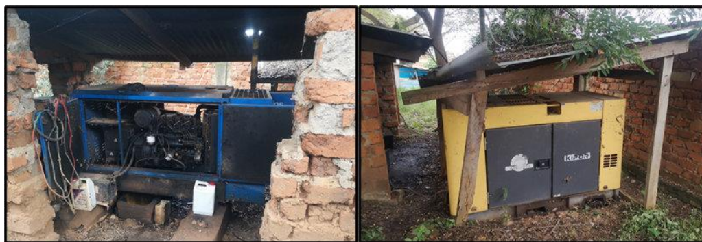
Figure 5-1. Generators observed on the project camp, May 2021.
