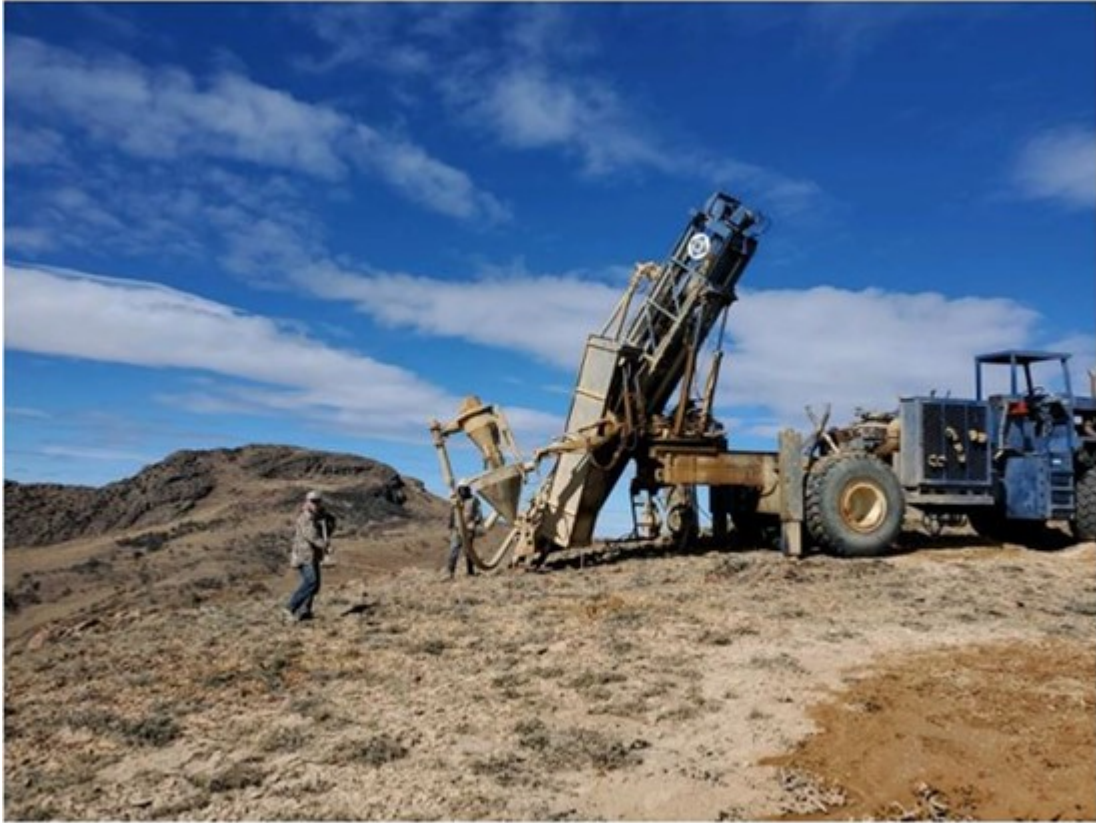
Figure 1 - Drilling hole 45 into the feeder structure. White Rock Mountain in the background. Next year's drilling plans to extend the gold zone into White Rock Mountain.
