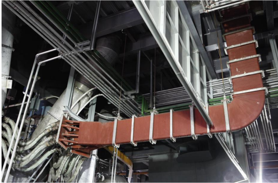
Figure 80: Typical Picture of the Bus Tube System used for Three Single-Phase Transformers
