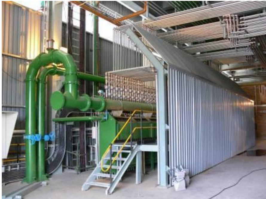
Figure 78: Furnace Cooling Water Supply Header and Tundish and Small-Bore Piping
