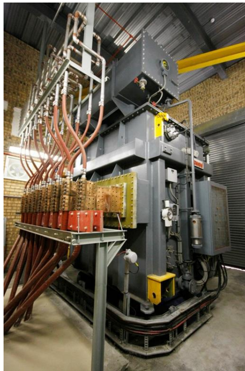
Figure 79: Typical Furnace Transformer
