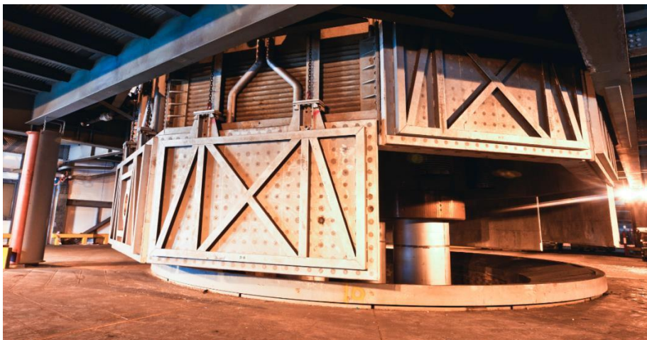
Figure 64: Furnace Smoke Hood
