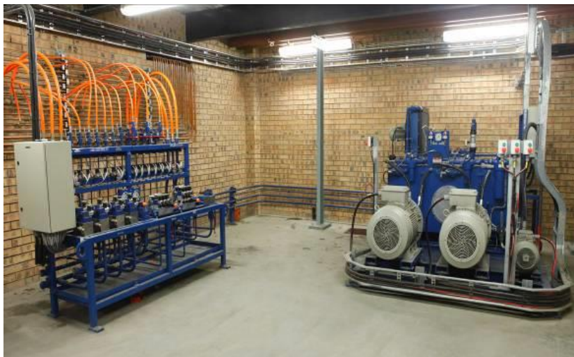
Figure 77: Furnace Hydraulic System by Tenova
