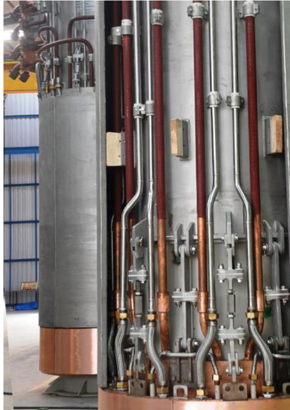
Figure 73: Electrode Heat Shield and Risers designed and supplied by Tenova
