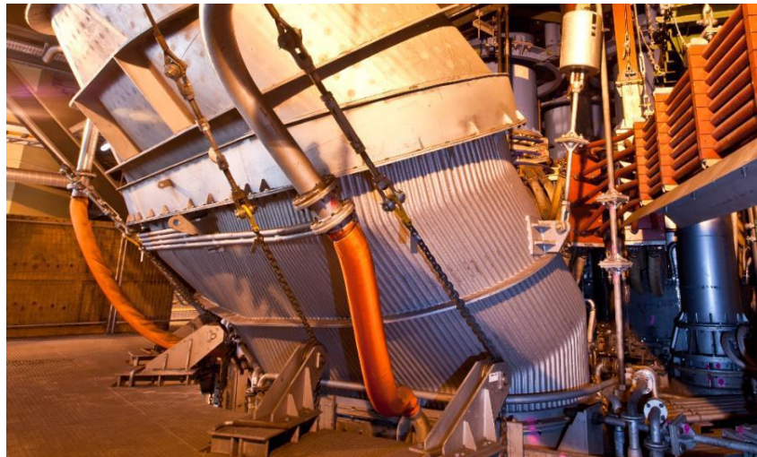
Figure 66: Furnace Off-Gas System designed by Tenova
