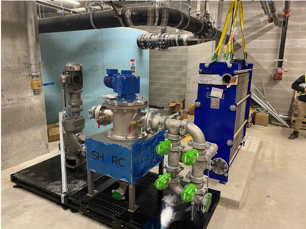
Pictured above: A SHARC WET System installed at Ielam
