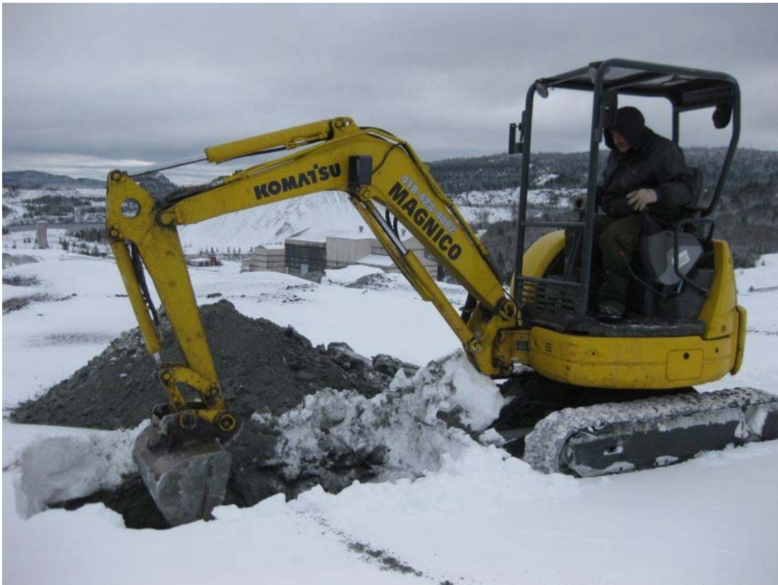
Figure 11.1: Test pit excavation on upper surface of Tailings. Mine site infrastructure in background.
