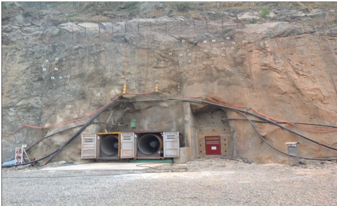
Figure 16-25: Akoti 2x315kw Exhaust Swedvent Fans
