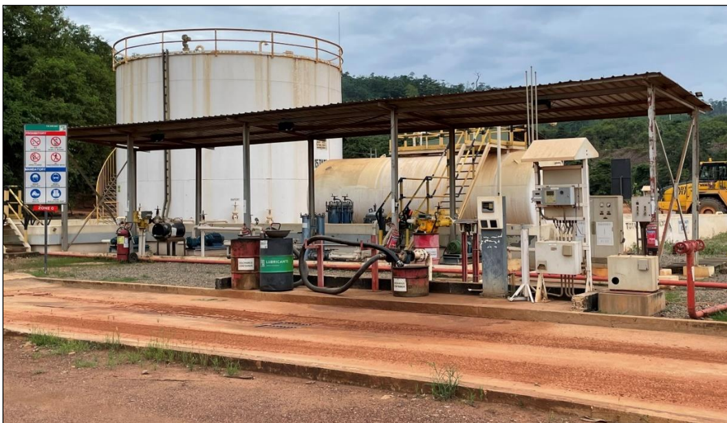
Figure 18-10: Fuel Farm at the Mine Services Area
