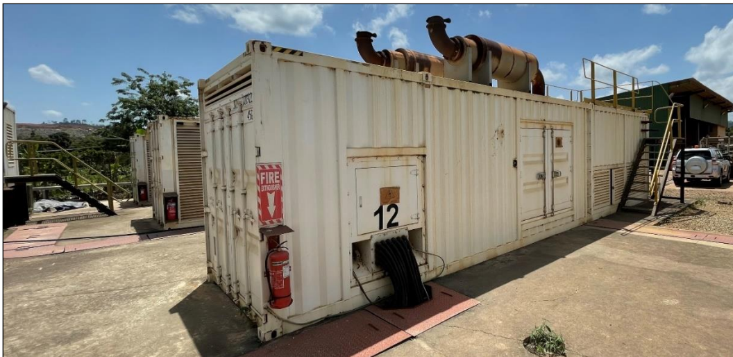
Figure 18-11: Gensets at the Processing Plant
