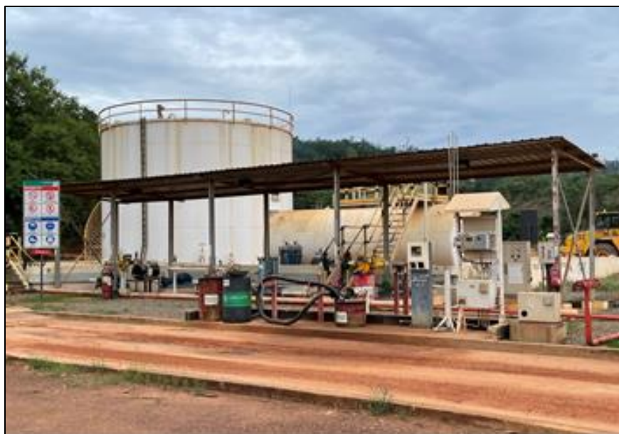
Figure 18-11: Fuel Farm at Mine Service Area
