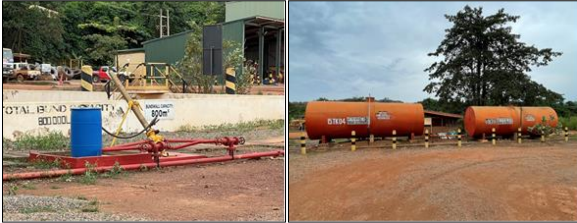
Figure 18-13: Fire Suppression System at Mine Service Area Fuel Farm
