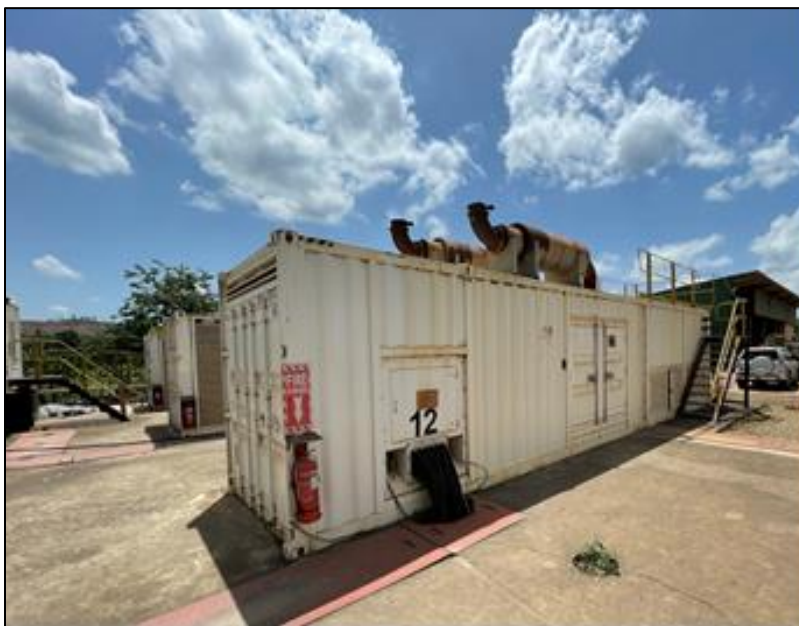
Figure 18-12: Gensets at Processing Plant
