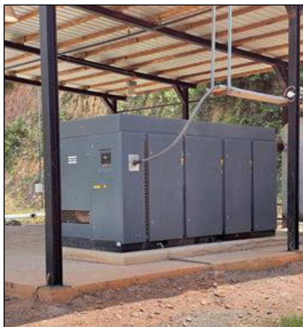
Figure 18-20: Compressor at Obra
