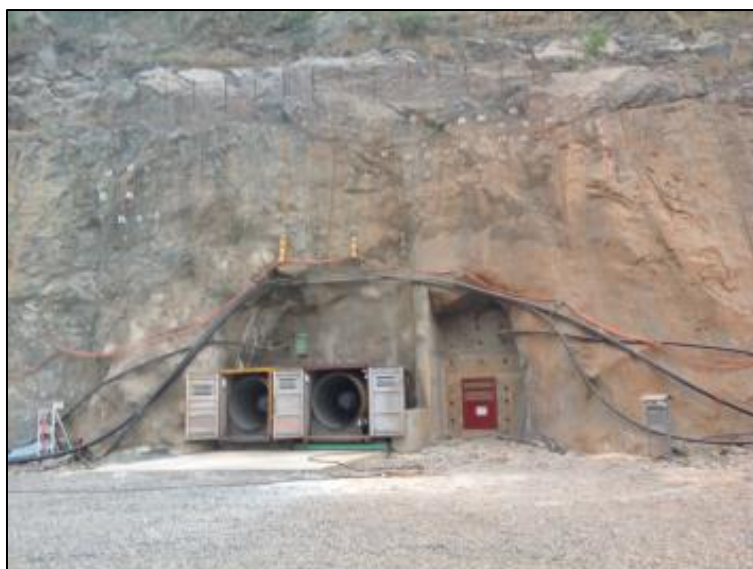
Figure 18-23: Swedvent Primary Ventilation Fans, Akoti Underground Mine
