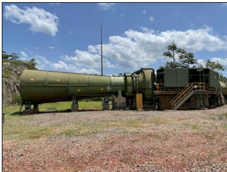
Figure 18-22: Howden Primary Ventilation Fans, Paboase Underground Mine
