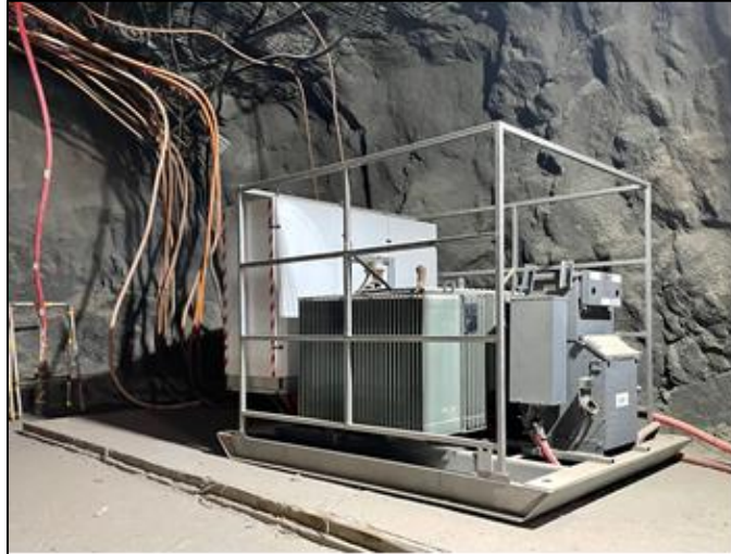
Figure 18-18: Underground Transformer at Suraw
