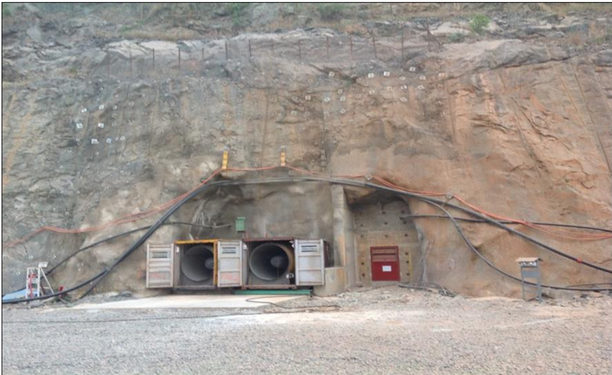
Figure 16-18: Akoti 2x315kw Exhaust Swedvent Fans
