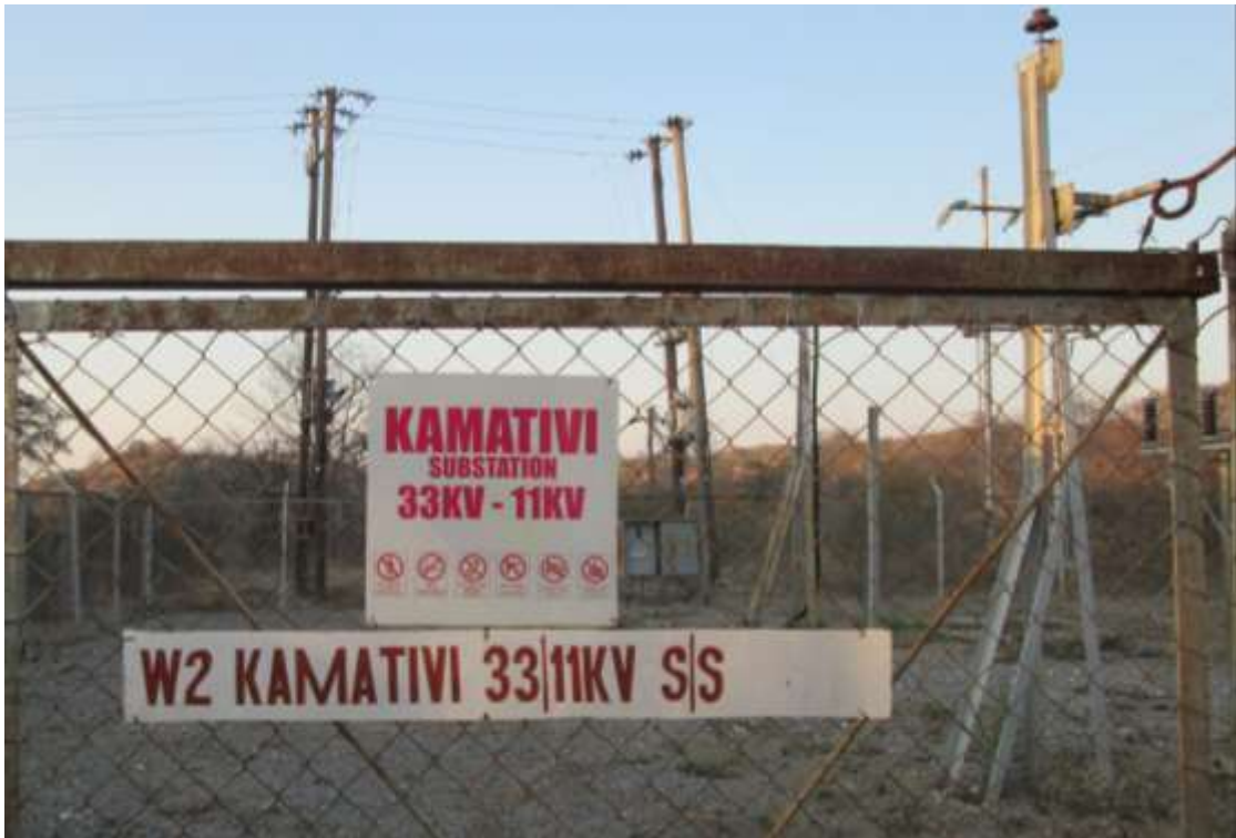
Figure 5-7 Kamativi Mine substation
