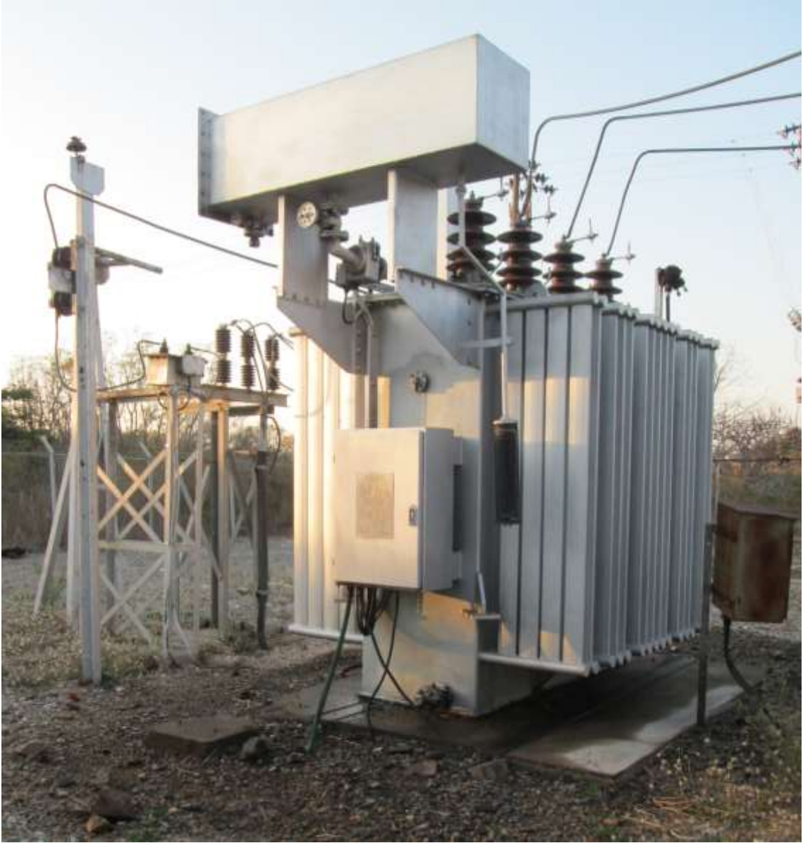
Figure 5-8 Kamativi Mine transformer
