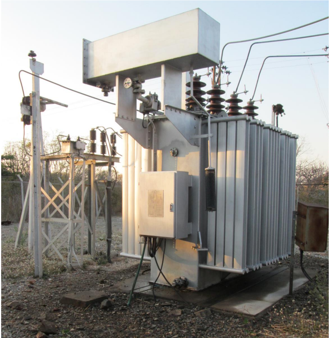
Figure 5-8 Kamativi Mine transformer
