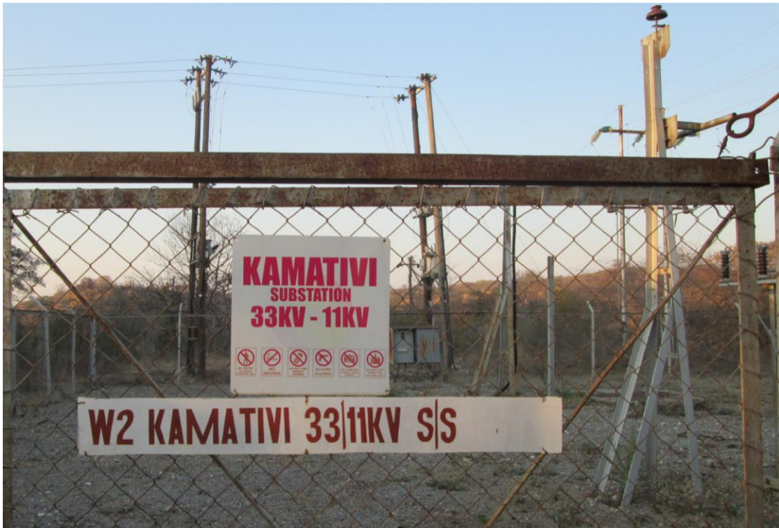
Figure 5-7 Kamativi Mine substation
