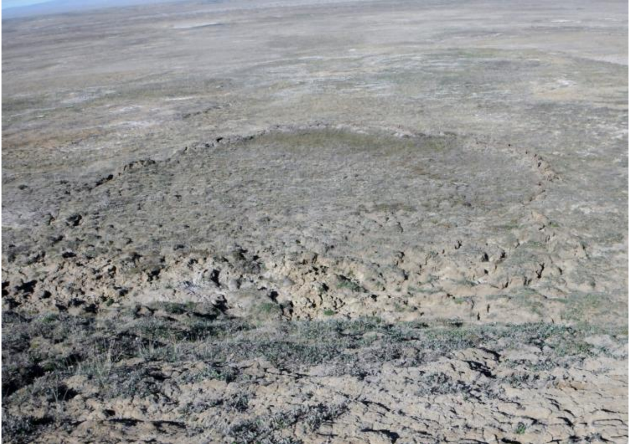
Figure 12.10: Slump on western side of runway area. Picture was taken from above, at the edge of the runway surface.
