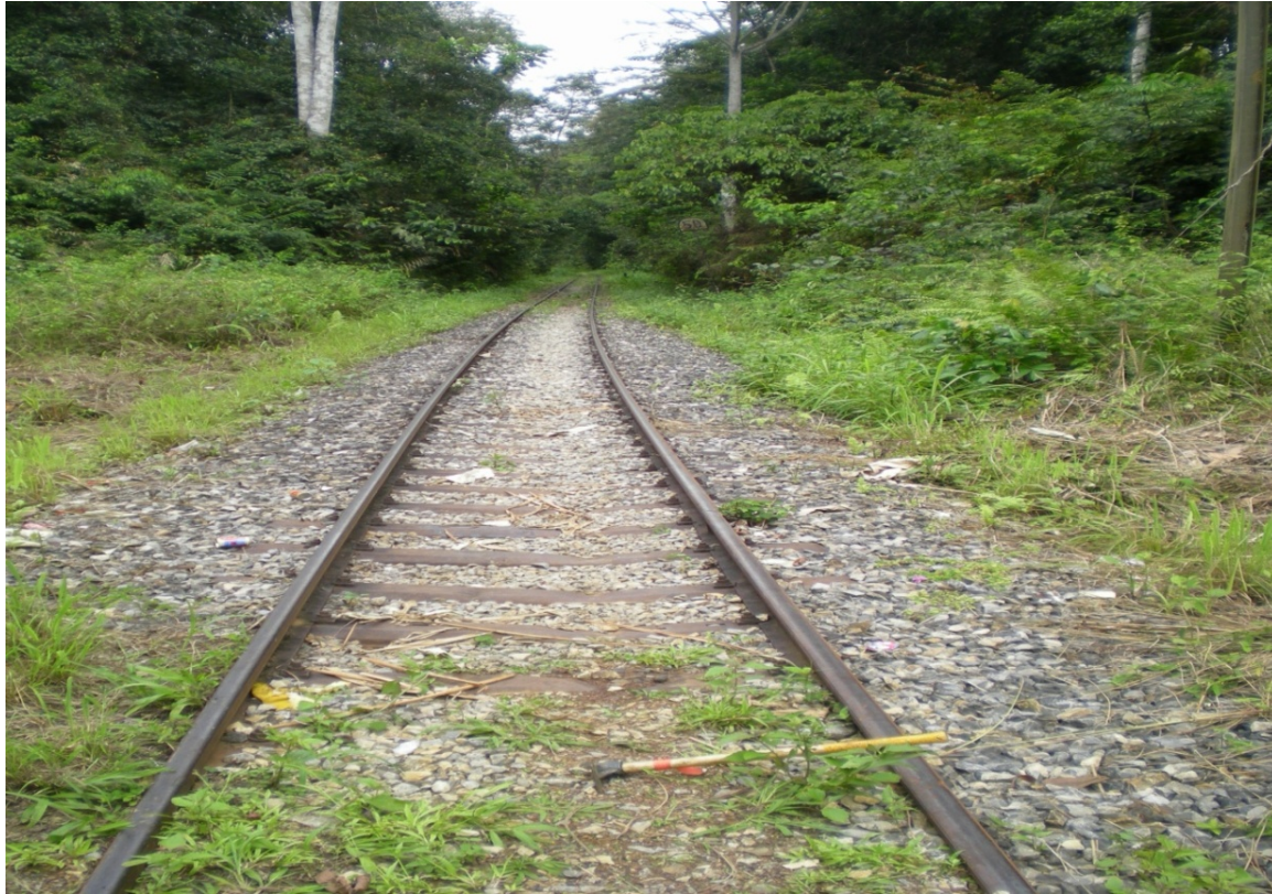
Picture 4: A view of the Camilog “Cape Gauge” narrow gauge railway. Note the steel sleepers dating from 1976 and the approximately 70 lb/yard rails, inadequate for the anticipated transport of iron ore.
