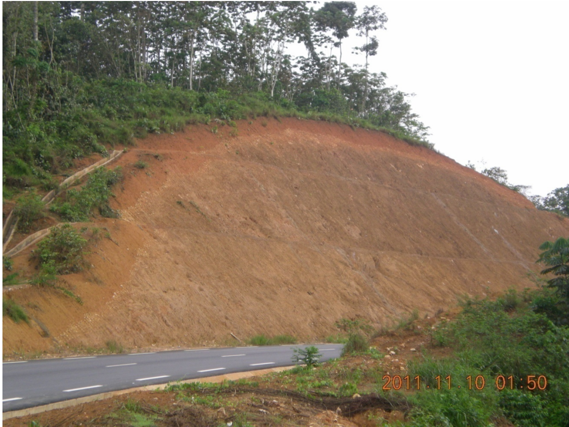
Picture 9: A view of a road cut along the Pointe-Noire - Brazzaville N-1 highway through the Mayombe mountain range. The bedrock is a completely laterized schist or gneiss. Note the 1-2 m thick zone of bioturbation at the surface (ochre layer) and the underlying laterite, where the mud has preserved the ghost structures of the original rock (foliation dips to the right).
