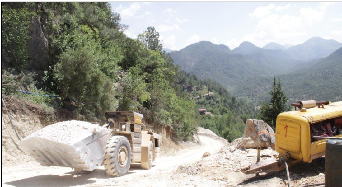
Figure 5: Pinargozu mine portal access road Showing typical mountainous terrain with extensive tree cover
