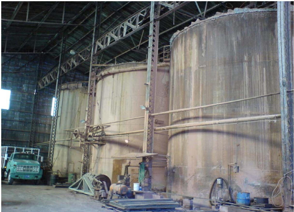
Figure 6.3 Atlanta Mill - Agitator tanks
