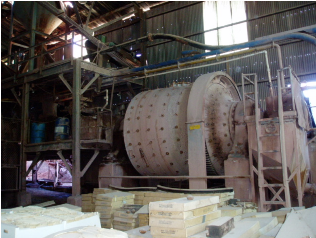
Figure 6.2 Atlanta Mill – Primary Ball Mill
