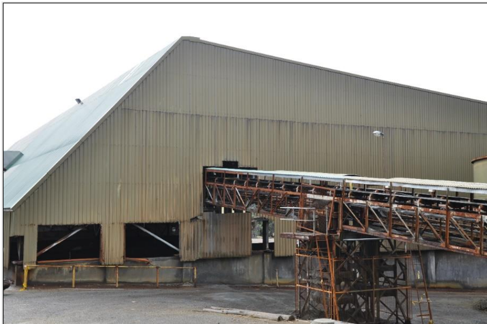
Figure 18-8. View of the concentrate shed from outside at the Bernie Port
