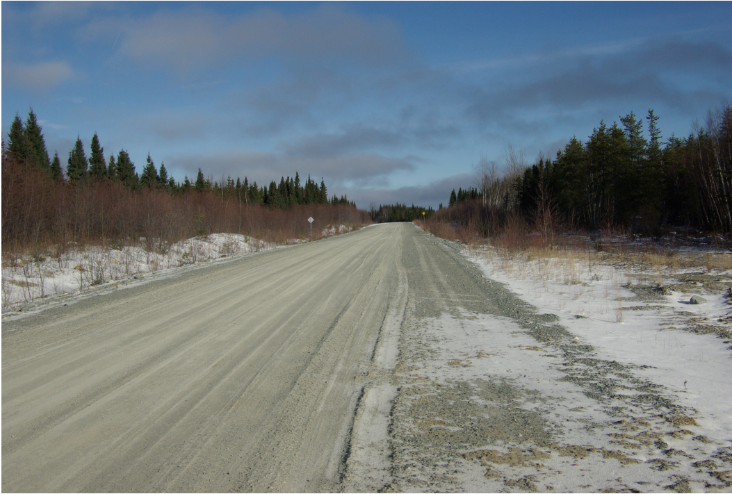
General view of road R1009, the main access road, open year round
