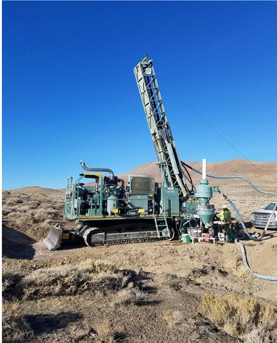
Figure 1 – MPD-1500 Drill Rig operated by DeLong working on the Rainbow Canyon Project
