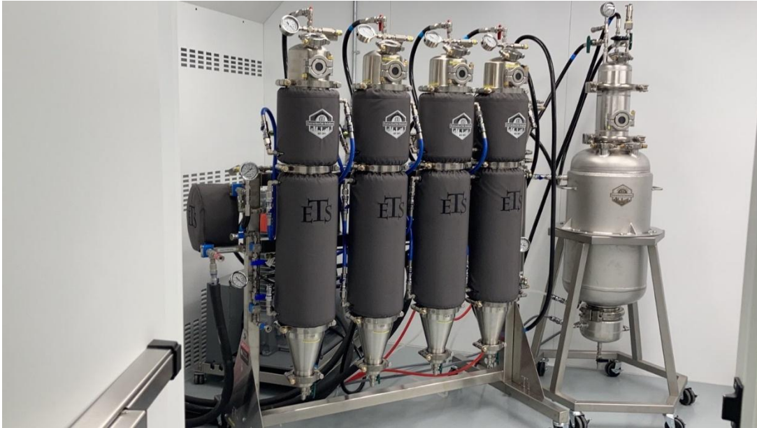
Figure 2 – ETS MeP™ XT70 Hydrocarbon Extractor assembly at Adastra Facility.
