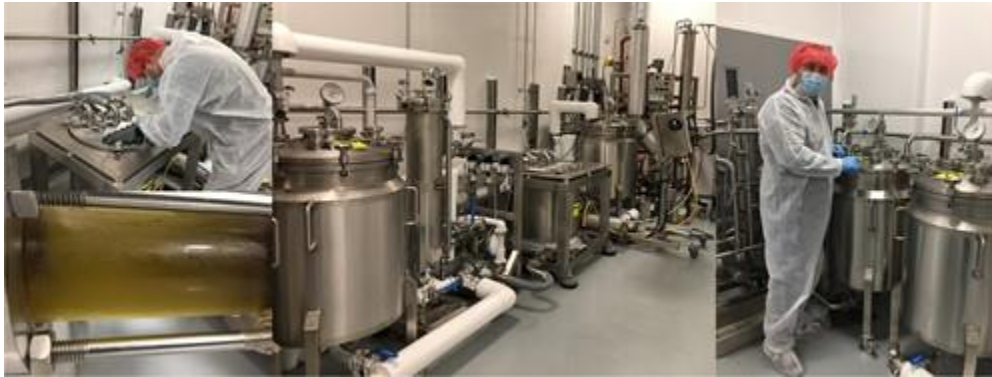
Figure 1 - Commissioned Cryo-Ethanol Extraction System in Adastra
