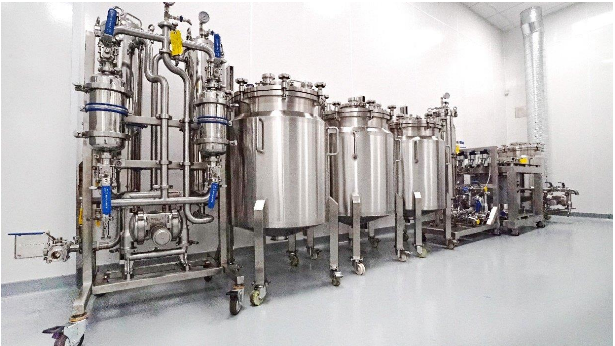
Figure 2 - EV-MASS Cryo-Ethanol System in Adastra Facility
