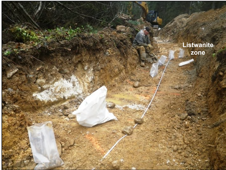
Photo 1: TR19-02, view looking westerly (J. Pautler, October 21, 2019)
