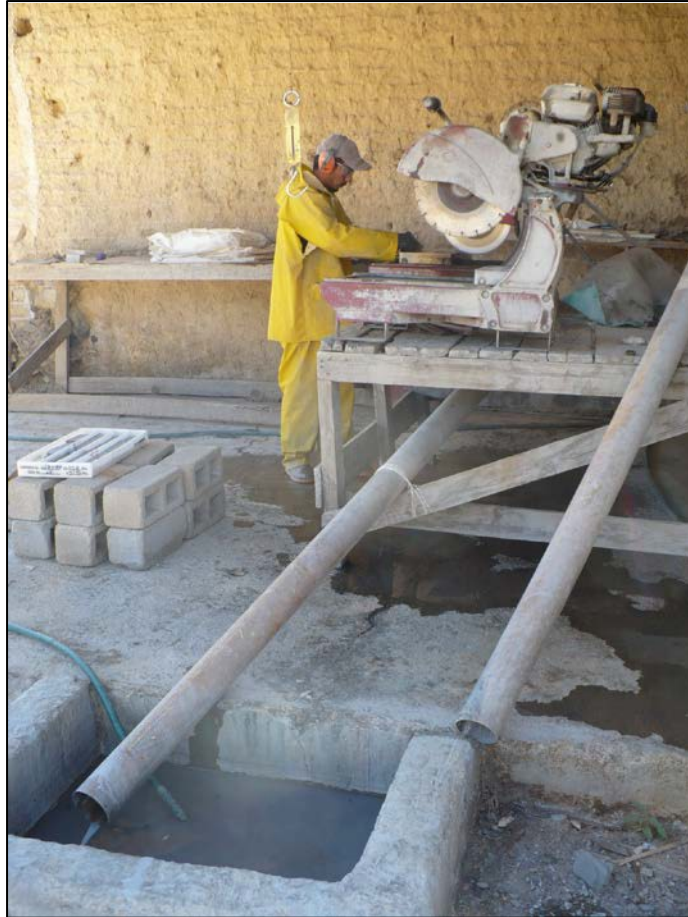
Figure 11-1: Core Cutting and sample prep area at core logging / core storage facility
