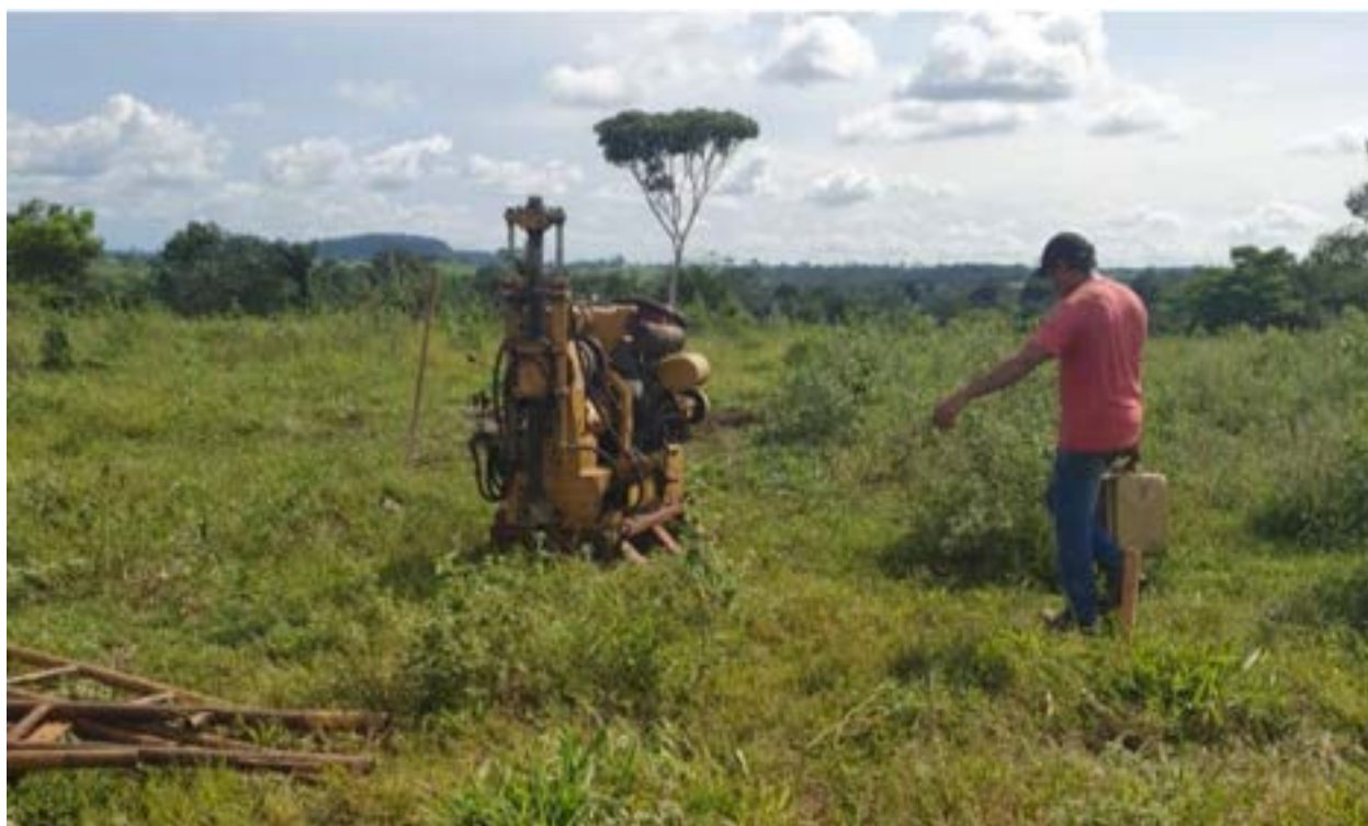
Figure 10.2 Photo of the SR-001 drill pad and the 27 hp Maquesonda 850 drill rig employed by Georrás to execute drill holes SR-001 and SR-003.
