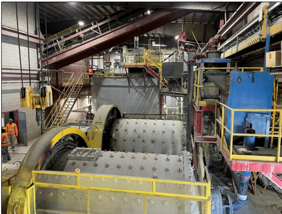
Figure 1: Photo of interior of Beacon Mill currently undergoing detailed inspections for restart
