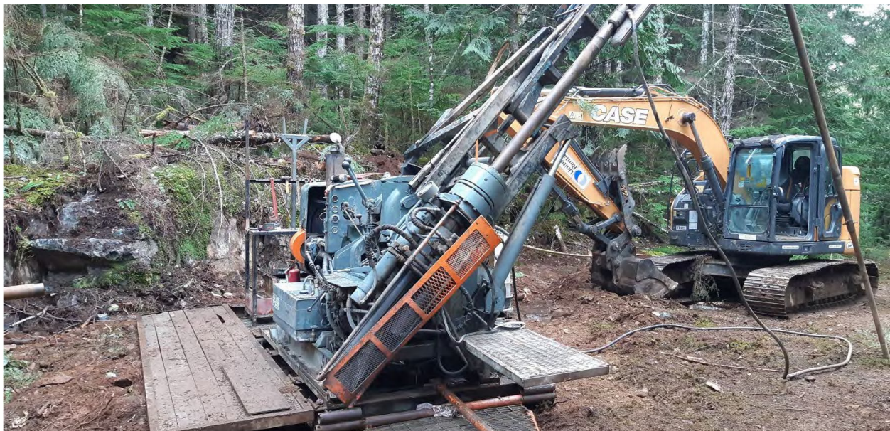
Figure 1 – Boyles 25 Diamond Drill on Setup #1 during previous drill campaign at Redonda Copper Project
